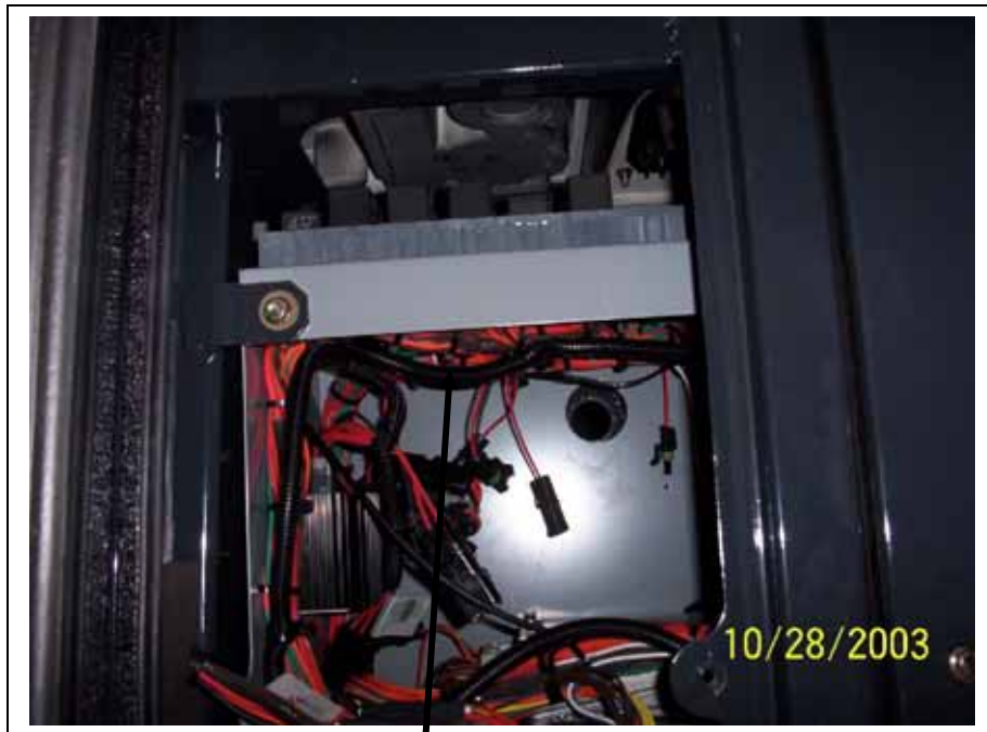
Clutch wire with loom re-installed running up the wire bundle towards the thermostat.
