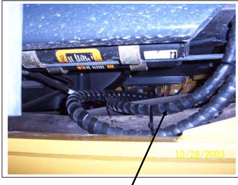
5/16" and 1/2" hoses under the cab looping up towards the existing knockouts in the cab floor on the left side of the cab.
