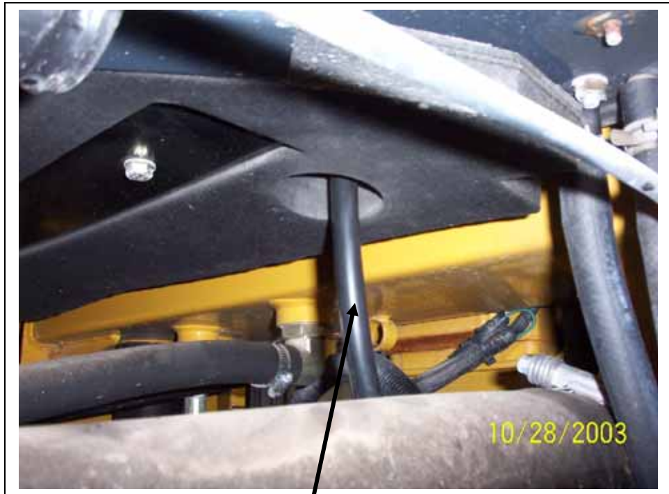
5/16" line connected to the expansion valve.
